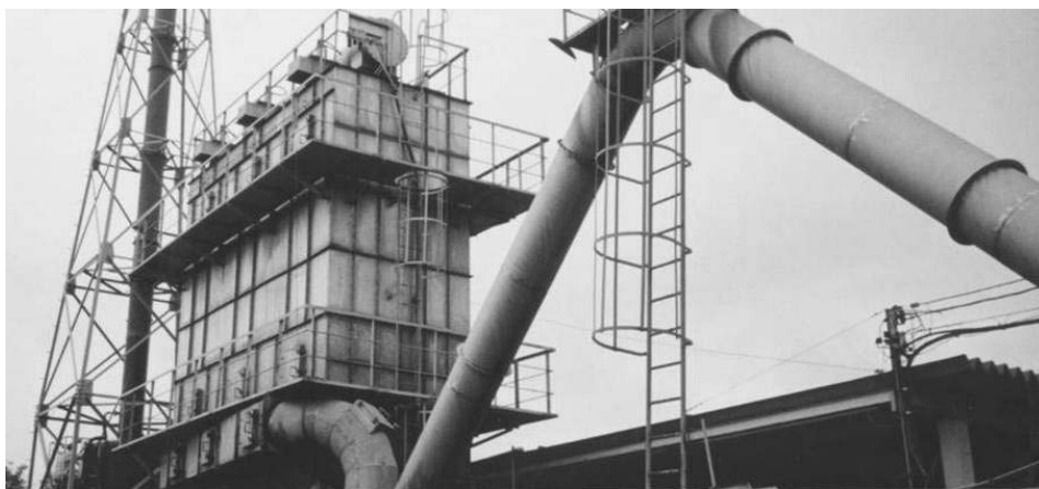
Pollution Control Facilities in Lead Recycling Plant in Japan. Photo by Michikazu KOJIMA
